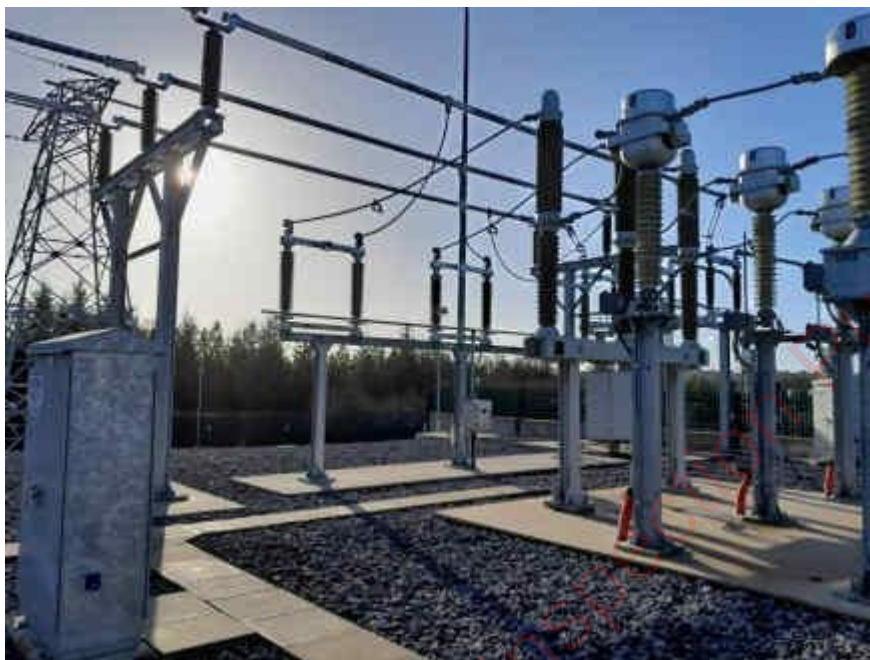
Plate 2-3 Typical 110kV electrical infrastructure
