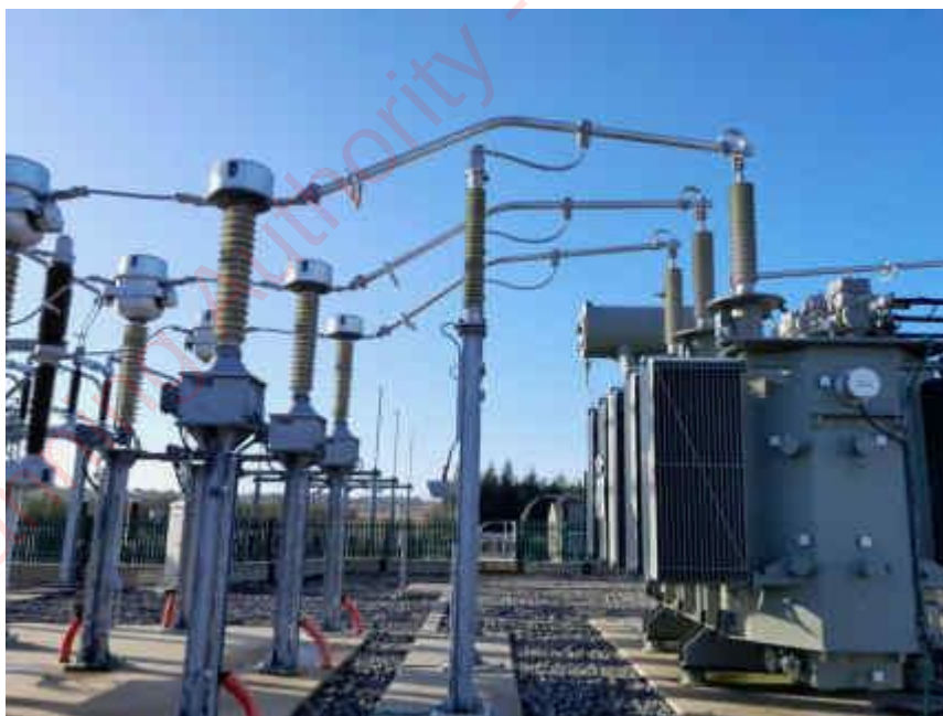
Plate 2-4 Typical 110kV transformer connection
