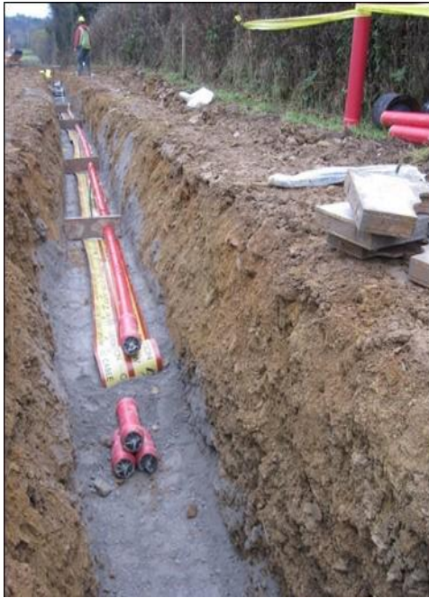
Plate 2-2 Typical Trefoil Cable Trench View
